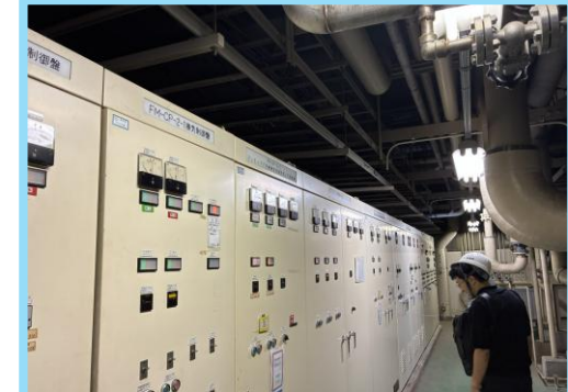
Control panel located on-site
