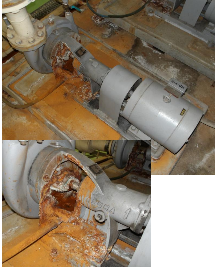
Low power pump for HVAC
