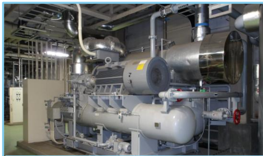
Screw Chiller (~400 kW) * Vacuum chamber and HVAC
