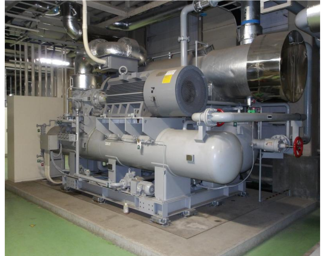
Screw chiller (~400kW)
