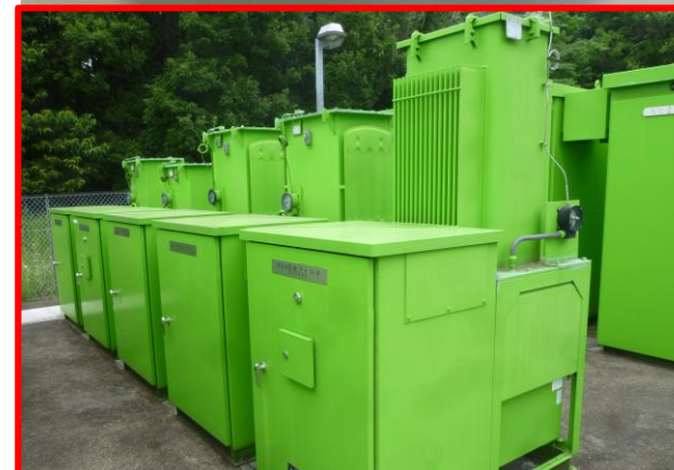
High Voltage Phase Advance Capacitors High Voltage harmonic filters * Linked to the control of the APFC.
