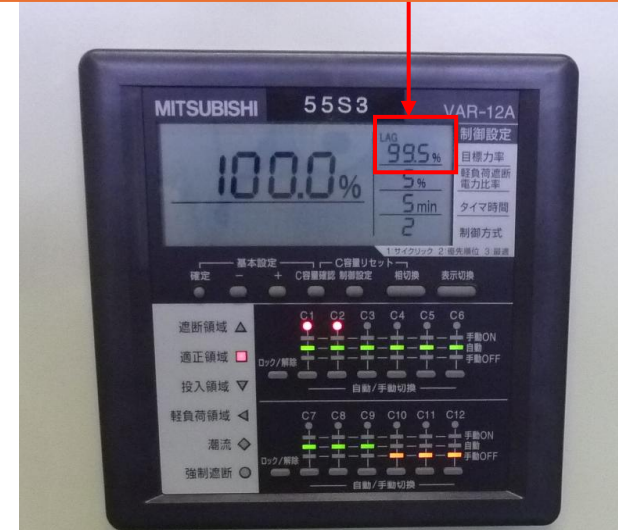
Automatic Power Factor Controller (APFC)
