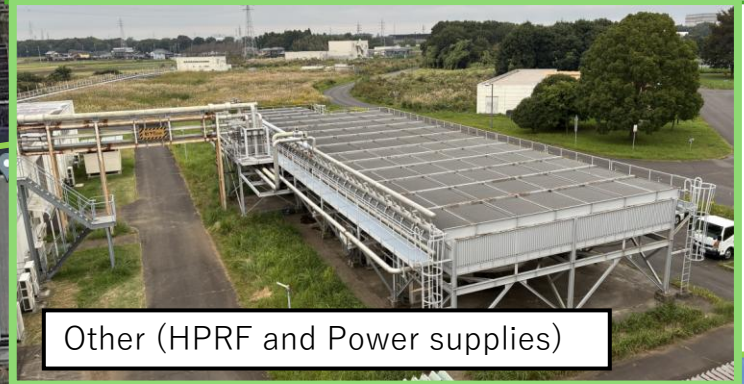
Air-cooled heat exchangers for the various devices
