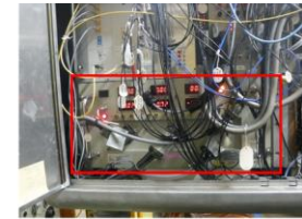
NIM-POWER SUPPLY Unit in GU_AT HV-ST
