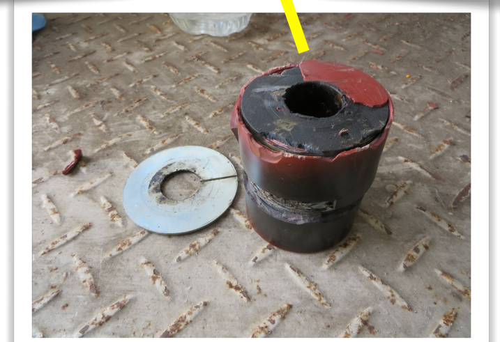
Broken solenoid coil of compressor-related valve
