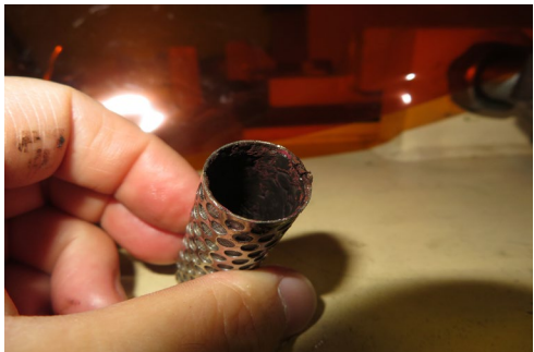
Strainer undergoing maintenance. It is clogged with copper oxide.
