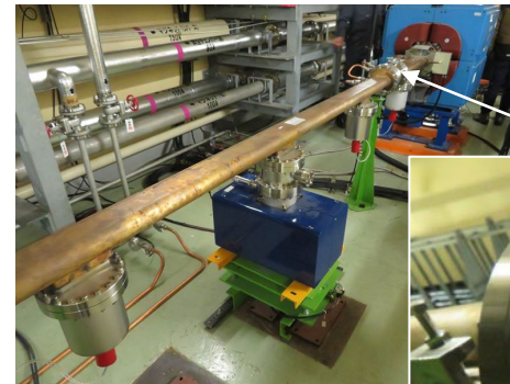
Leaked bellows chamber
