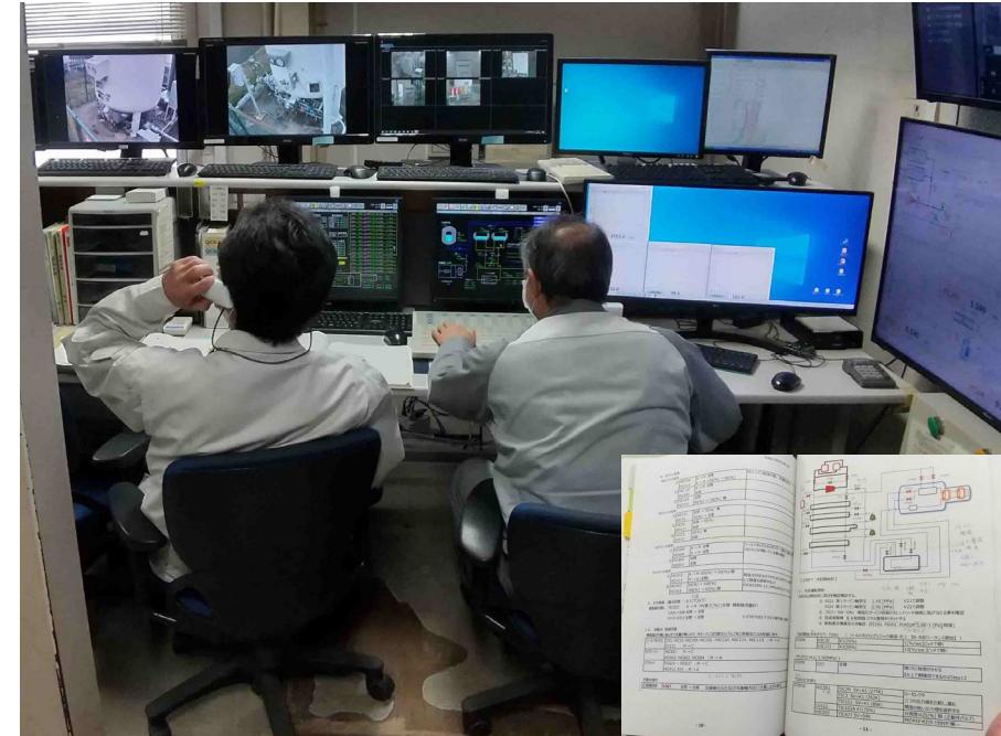
Nikko control room
